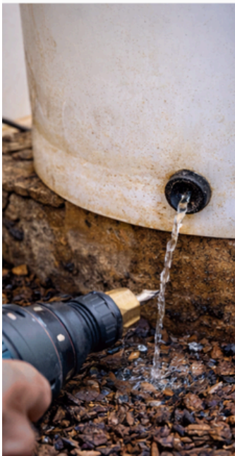
Hole drilled too low → sediment clogs fitting
